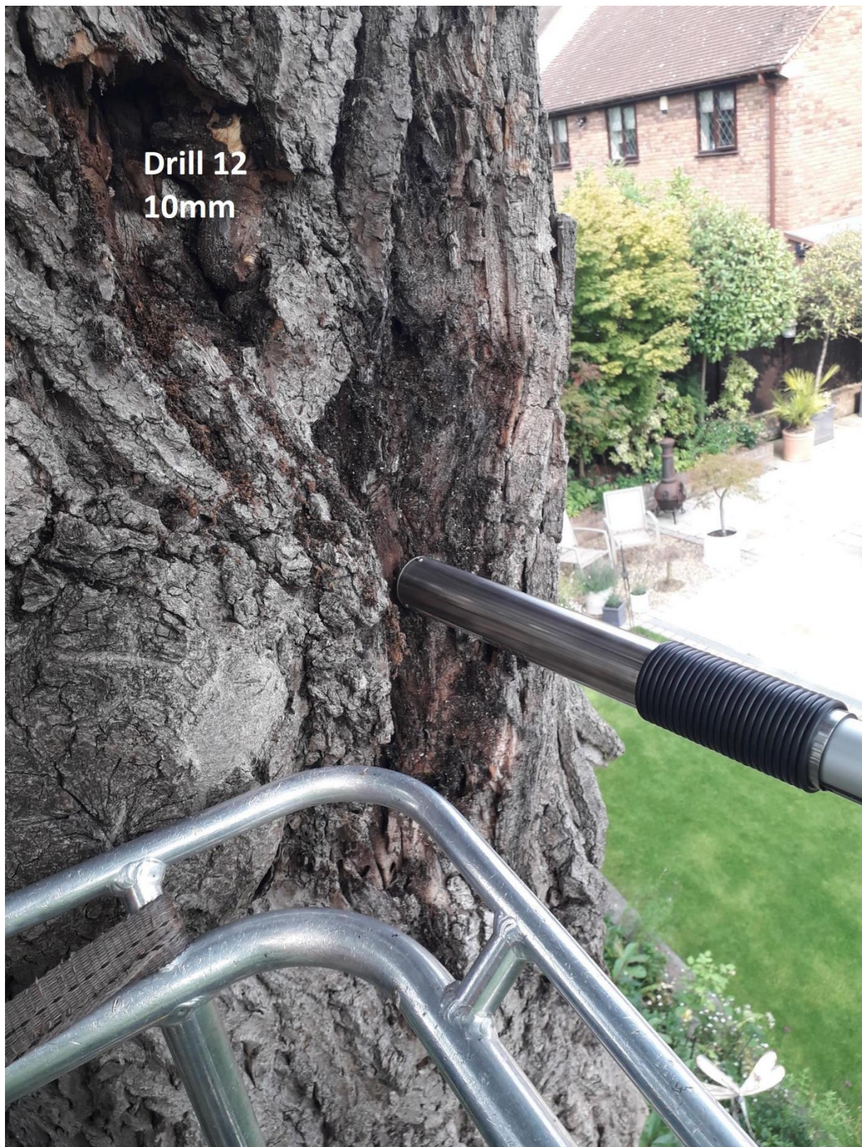
Photo 12 – drilling 12. Large area of bark killing and thin layer of new wood.
