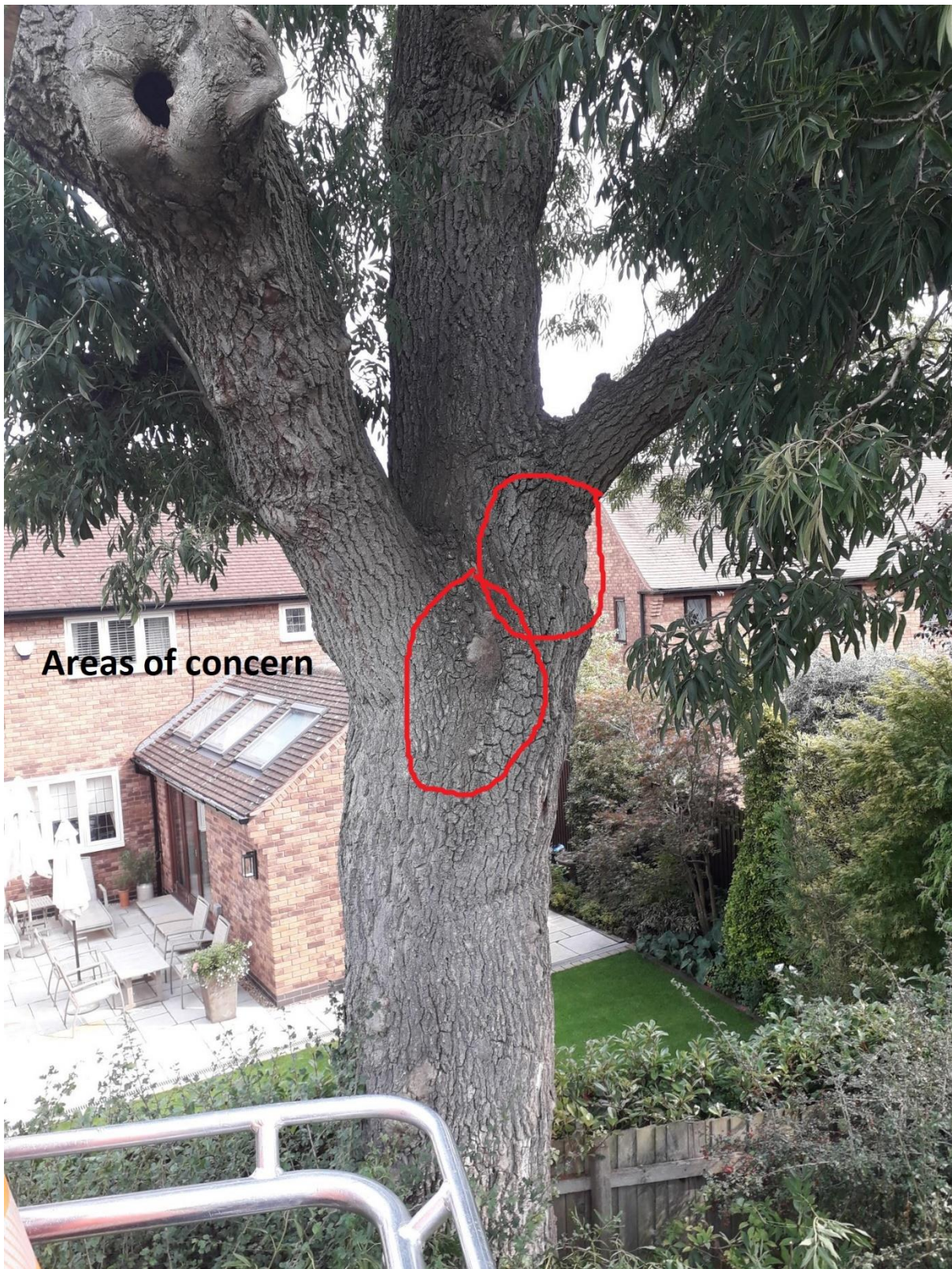
Photo 13 – areas of concern. Mid trunk. Drilling 7 to 10.
